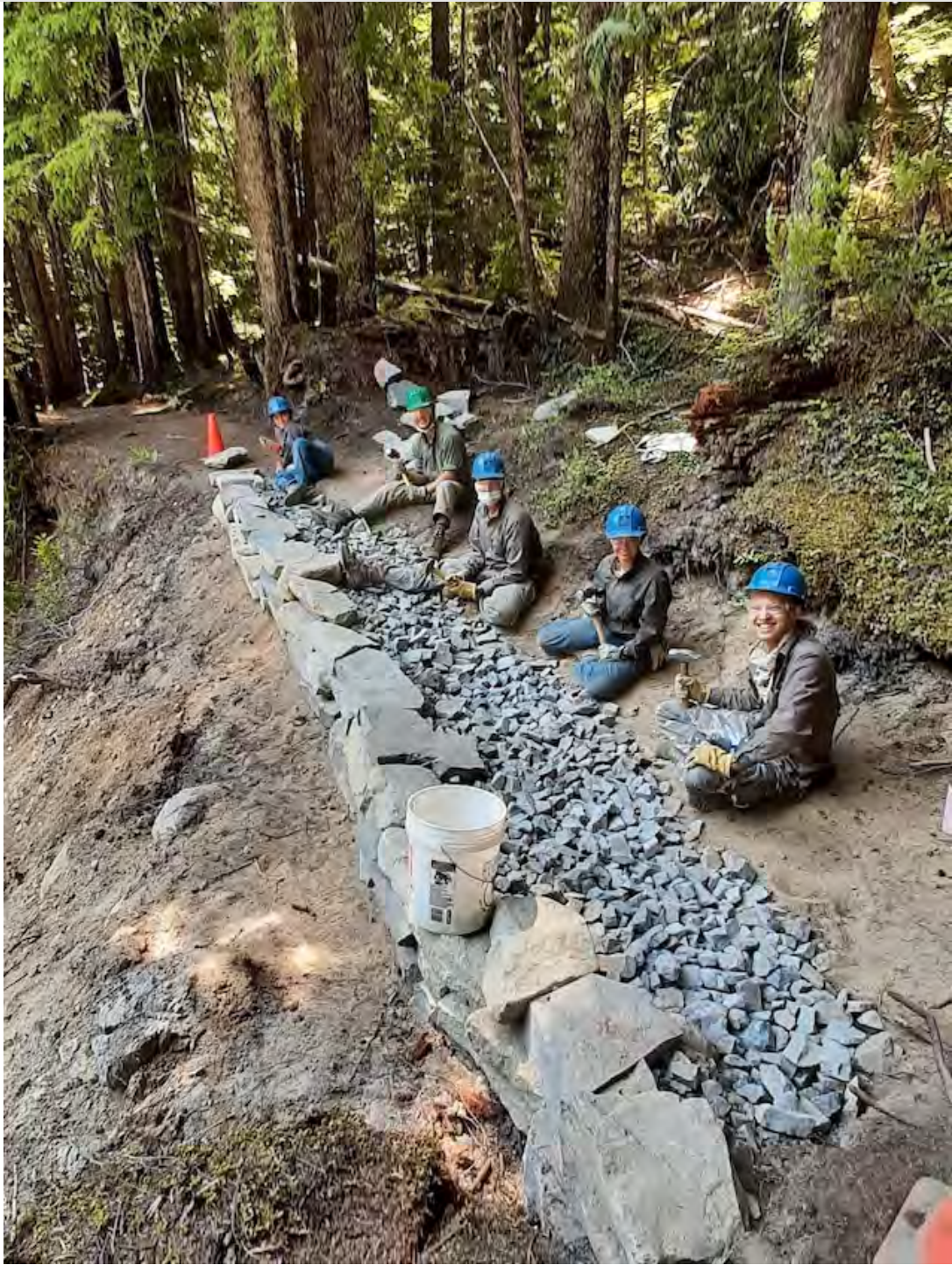
Members of the Rainbow Crew construct a stone retaining wall to provide trail stability at Mount Rainier National Park. COURTESY NORTHWEST YOUTH CORPS
