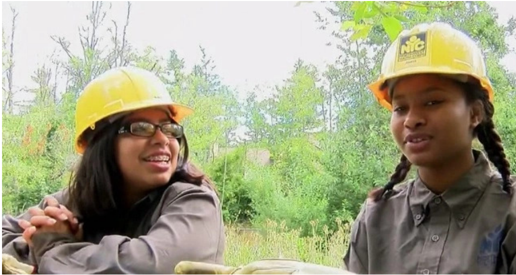
A group of 10 teenage girls are working together to repair a Troutdale bridge damaged in the high water late last year, July 26, 2016 (KOIN)
