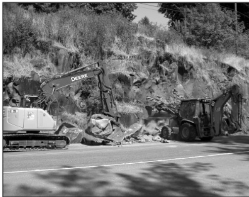
WALTERVILLE: With an eye toward upcoming winter storms, ODOT workers were busy this week next to the westbound lane's shoulder near milepost 18 of Hwy. 126. Excavators removed several tons of material from a rock wall prone to sloughing off large chunks during storm events.
